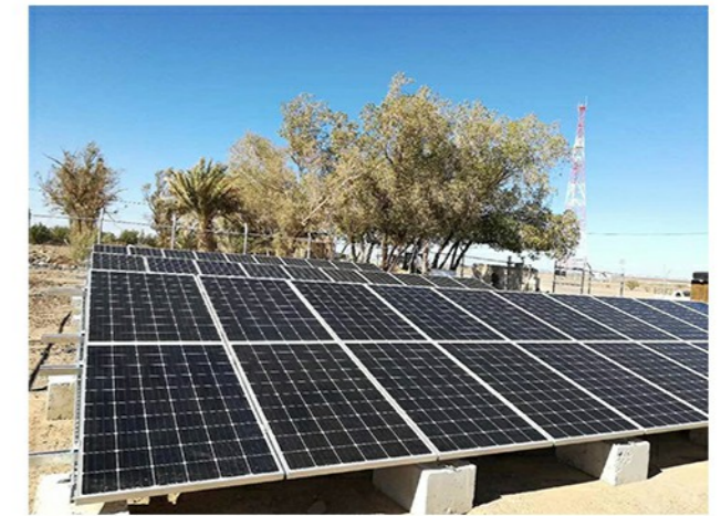
11KW Solar Irrigation in Saudi Arabia
