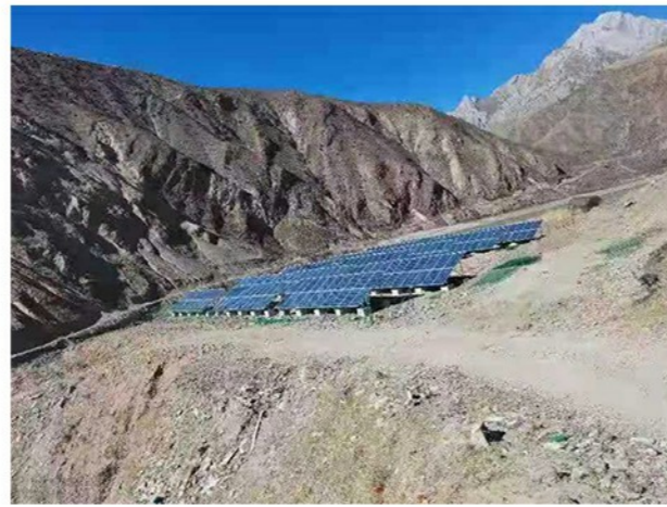
222KW Solar Pumping System in Sichuan Province
