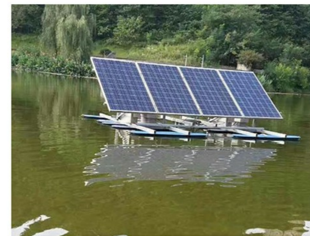
Solar Oxygenation System in Kunming
