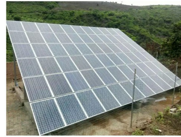
Solar Orchard Irrigation System in Yunnan Province
